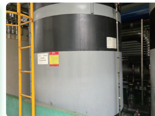
Collection of Recovered Water in a Tank for Reuse
