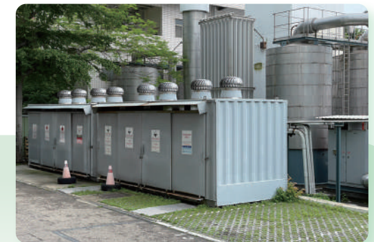
Temporary Storage Site of Hazardous Industrial Waste
