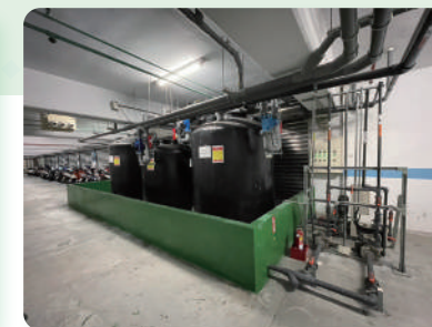
Collection of Process Wastewater
